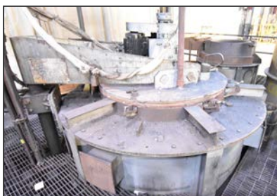
View of CUSTOM MFG pit draw furnace
