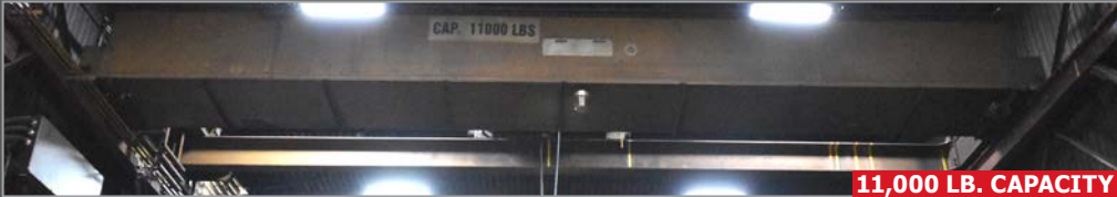
DEMAG overhead bridge crane
