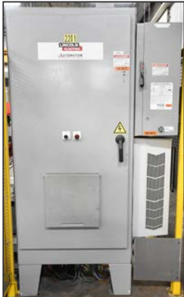
LINCOLN ELECTRIC/ALLEN BRADLEY PLC panel
