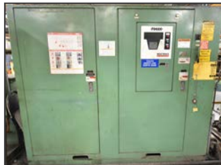
View of PLC panel
