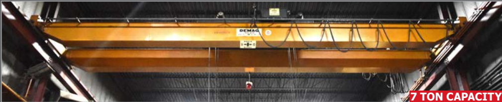
DEMAG overhead bridge crane
