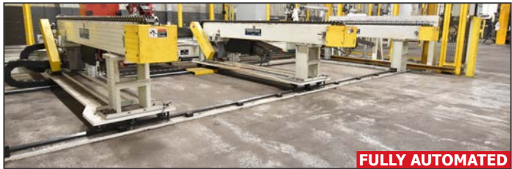
View of bar loading/unloading conveyors
