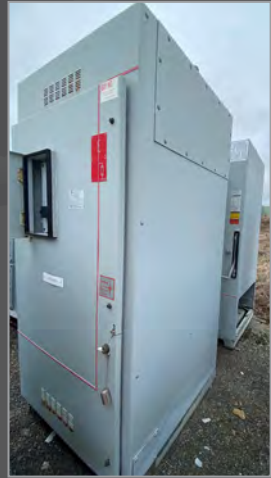
S&C electric switchgear units with 600A bus
