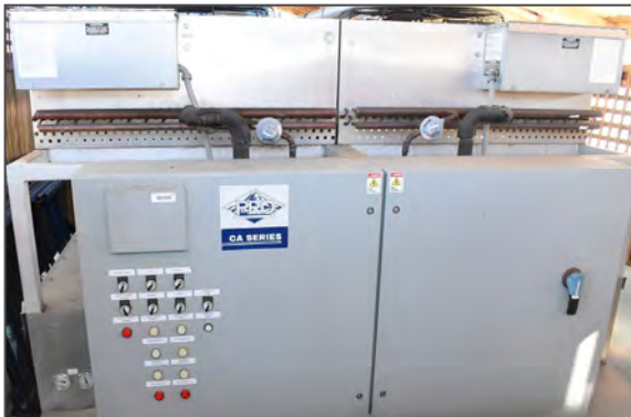
PRO CHILLER SYSTEMS CA SERIES MODEL RDS022EB2B12A1A glycol chiller
