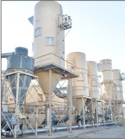
Partial view of dust collection system
