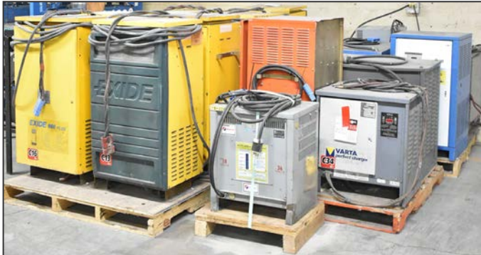
Partial view of forklift battery chargers available
