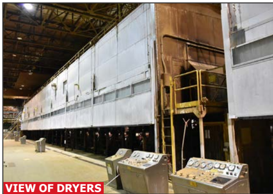
VIEW OF DRYERS
