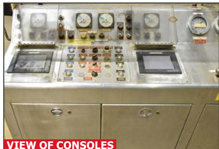
VIEW OF CONSOLES
