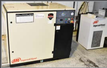
INGERSOLL RAND SSR UP6-30-125 rotary screw compressor & TS100 air dryer
