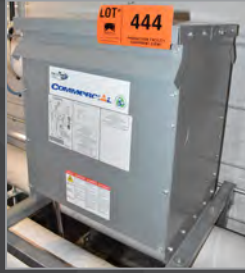
DELTA COMMERCIAL 30 KVA transformer
