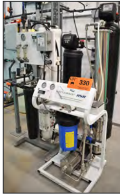
Commercial reverse osmosis water treatment system
