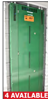
LEVITON lighting remote panel
