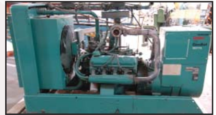
ONAN 75 KVA LPG standby generator
