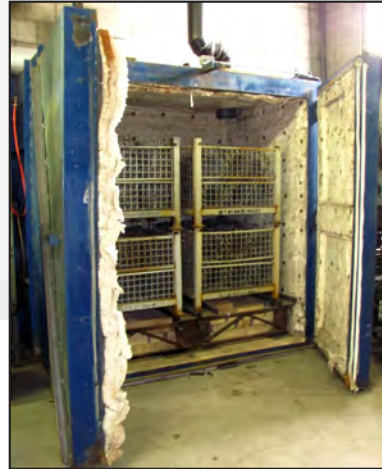
84" X 84" X 53" deep gas fired curing oven
