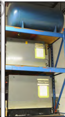
ATLAS COPCO GA 115 rotary screw air compressor & dryer
