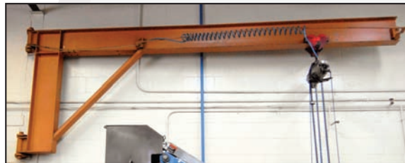
View of jib crane
