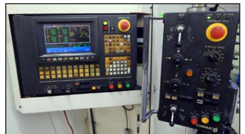
View of TOSNUC 888 CNC control panel
