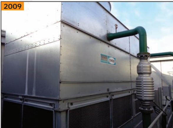
TOROMONT CIMCO cooling tower
