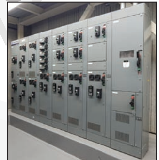
Partial view of switch gear available
