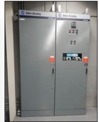
Partial view of switch gear available
